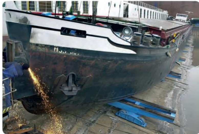
This inclined slide track, on which the heavy ship will glide into the water when it is launched, is painted with a special soap to reduce friction.
